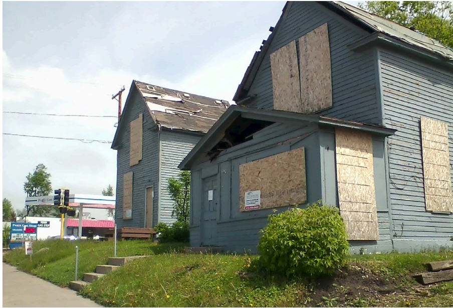
Figure 1. Condemned homes in North Minneapolis marked for demolition.
