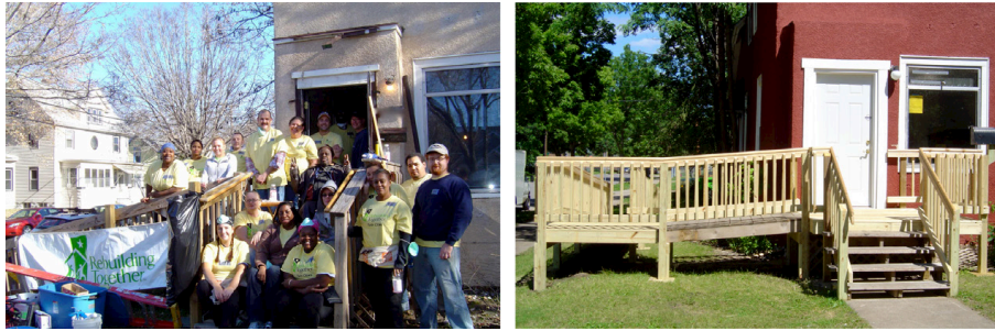
Figure 5. Accessibility ramp and exterior repairs for this low-income homeowner helped to make the home safer and more personal.
