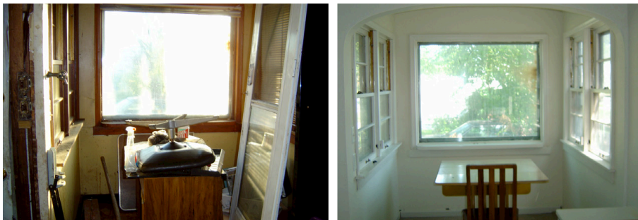
Figure 3. Repairs done by Rebuilding Together Twin Cities to create a workspace in the home of a low-income Minneapolis resident.
