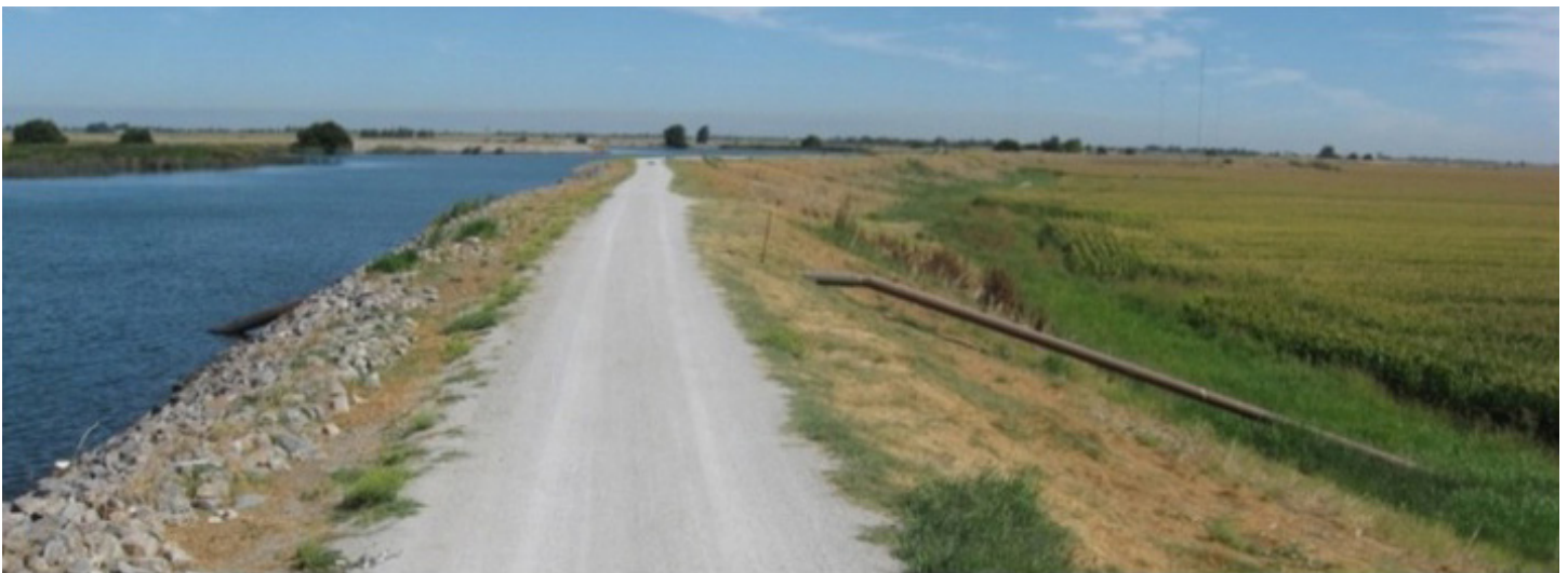
Figure 2 Subsidence on Staten Island, depicting a diversion siphon for scale
