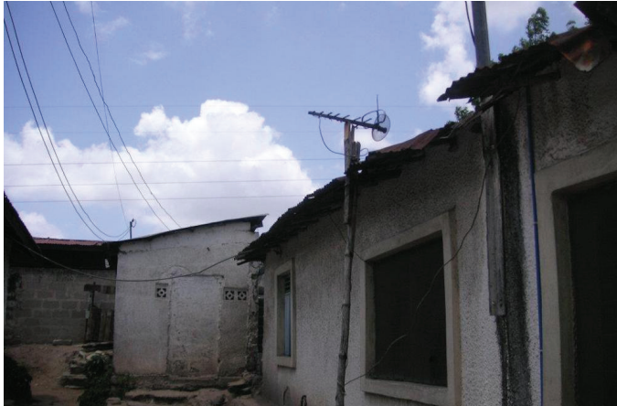
Service line wires dangle precariously over a secluded corner of Kibo. PHOTO BY MICHAEL DEGANI
