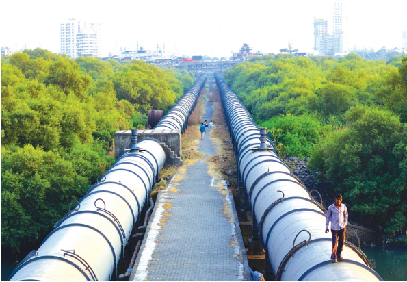
Mumbai's public water system, comprising more than 4,000 kilometers of pipe, has recently been the target of reform proposals that aim to improve supply. Nikhil Anand (p. 97) explores protest movements that advance a competing vision of the utility's "hydraulic public".
