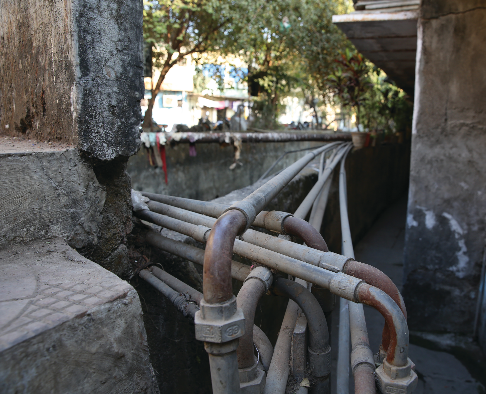
PIPE PUBLICS. A gathering of water service lines in Mumbai. (PHOTO: JESSE SHIPLEY)
