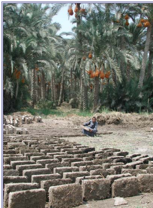
Figure 2. Striking new mud-brick. Note the earth-straw mixture in the background and brick turned for drying in the foreground.
