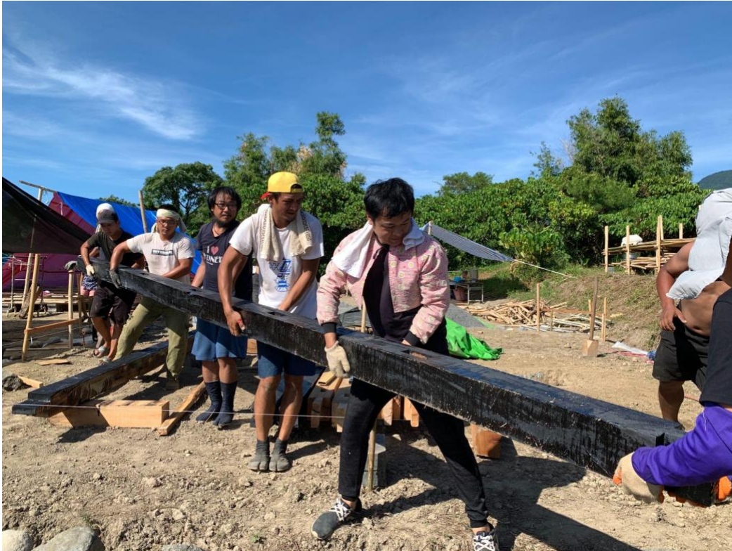
Figure 8. Volunteers working together in the construction of an Amis traditional house, Madawdaw, Taitung county, Taiwan, 2020. Photograph courtesy of Xie Song Zhi
