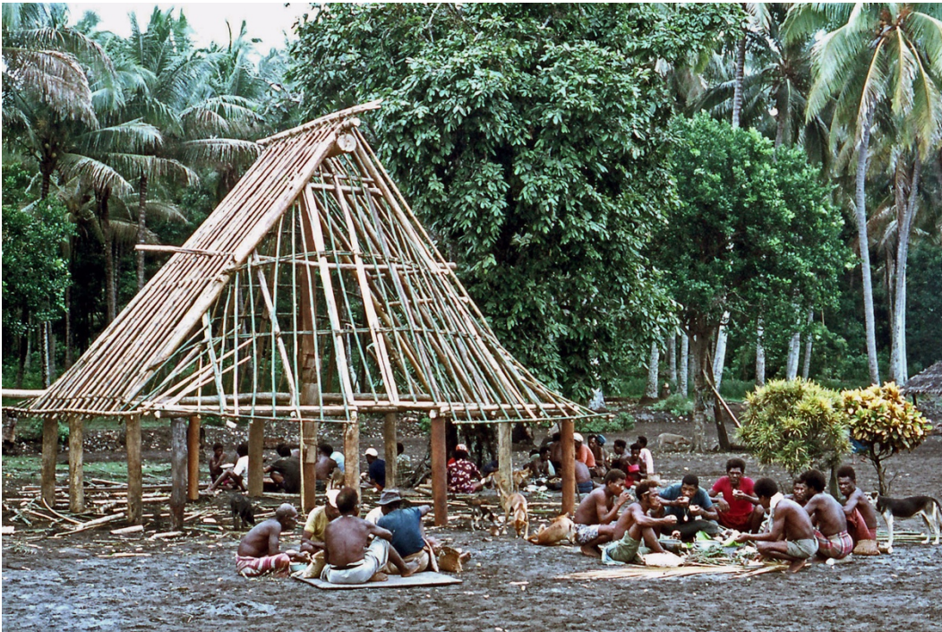
Figure 25. Having completed their work on the nalum for the day, the builders enjoy a meal sponsored by the local big man and prepared by Potne women. Potne village, Kilenge, West New Britain, Papua New Guinea, c. 1977. Photograph courtesy of the author
