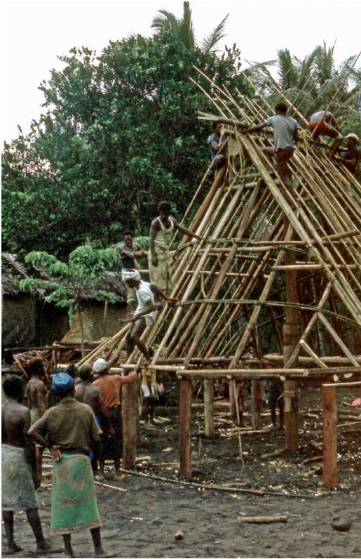
Fig. 24. Construction of the nalum roof. Potne village, Kilenge, West New Britain, Papua New Guinea, c. 1977. Photograph courtesy of the author
