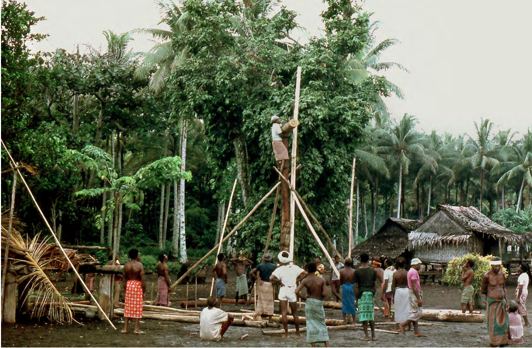
Figure 22. Construction of the naulum. Potne village, Kilenge, West New Britain, Papua New Guinea, c. 1977. Photograph courtesy of the author
