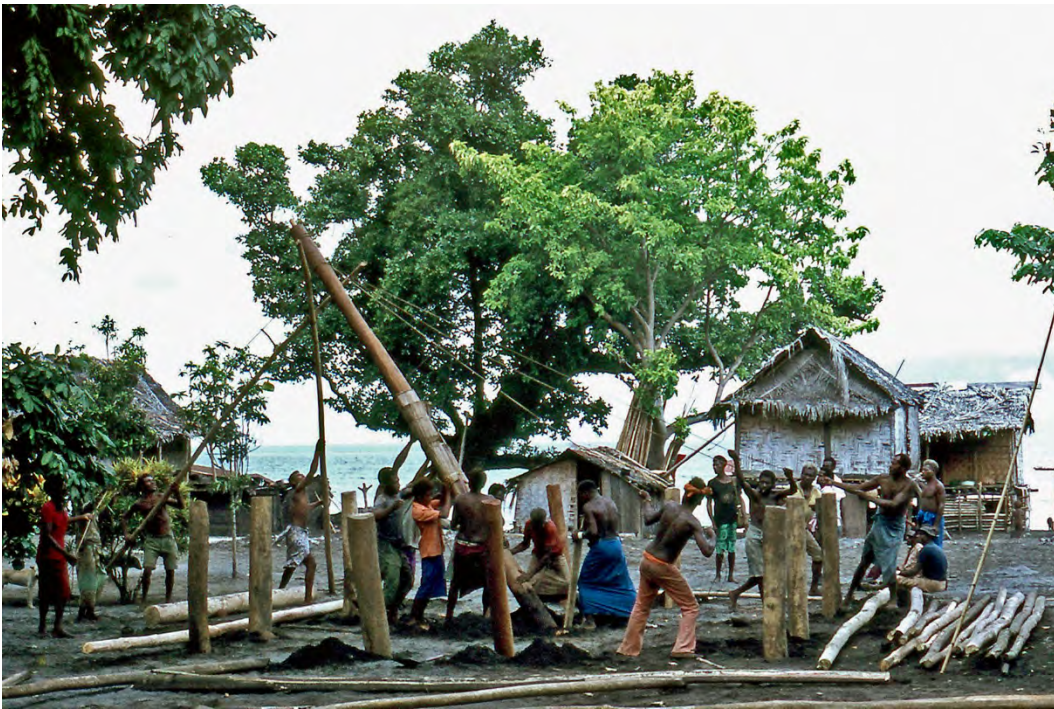
Figure 18. Erecting the central post of the naulum. Potne village, Kilenge, West New Britain, Papua New Guinea, c. 1977. Photograph courtesy of the author
