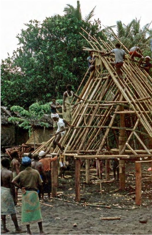
Fig. 24. Construction of the naulum roof. Potne village, Kilenge, West New Britain, Papua New Guinea, c. 1977. Photograph courtesy of the author
