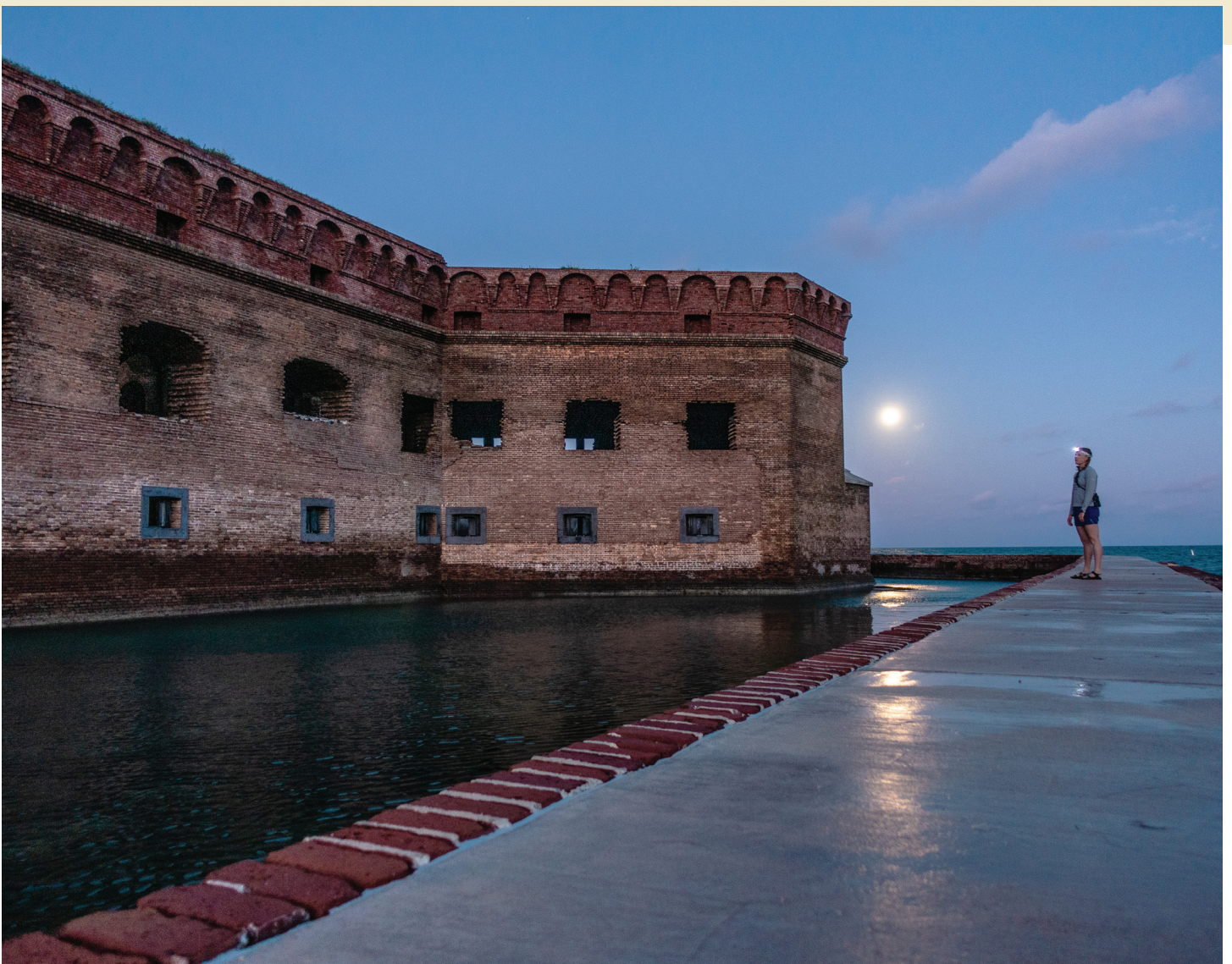
A visitor takes in the moonrise outside historic Fort Jefferson in Dry Tortugas National Park. This is one of the largest 19th-century American masonry fortifications. Sea level rise poses a significant threat to the fort. However, all seven islands of Dry Tortugas are under constant threat of inundation. Several of the islands disappear seasonally due to rising seas, including Middle Key. Bird Key has disappeared altogether. NATIONAL PARK SERVICE
