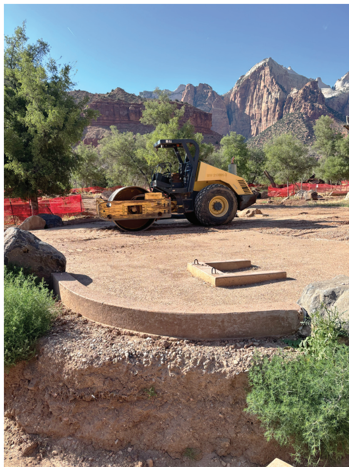
Sites under construction at South Campground in Zion National Park, photo taken from bike path through a fence opening.
