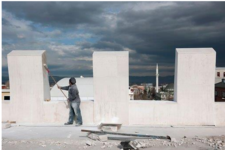
Fig. 8. A worker finishing up the stone façade on the rooftop of Argul Weave , which is now a restaurant, 2014. Photo credit: Thomas Mayer.
