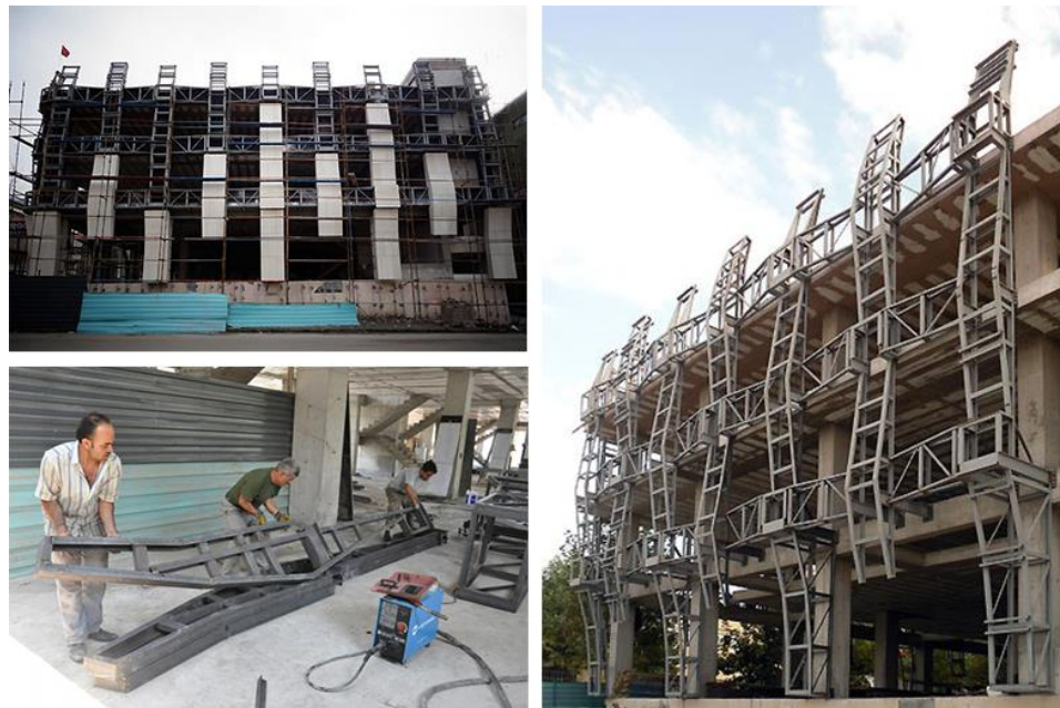
Fig. 7. Constructing the steel support for the signature stone façade of Argul Weave , 2014. Photo credit: Thomas Mayer.
