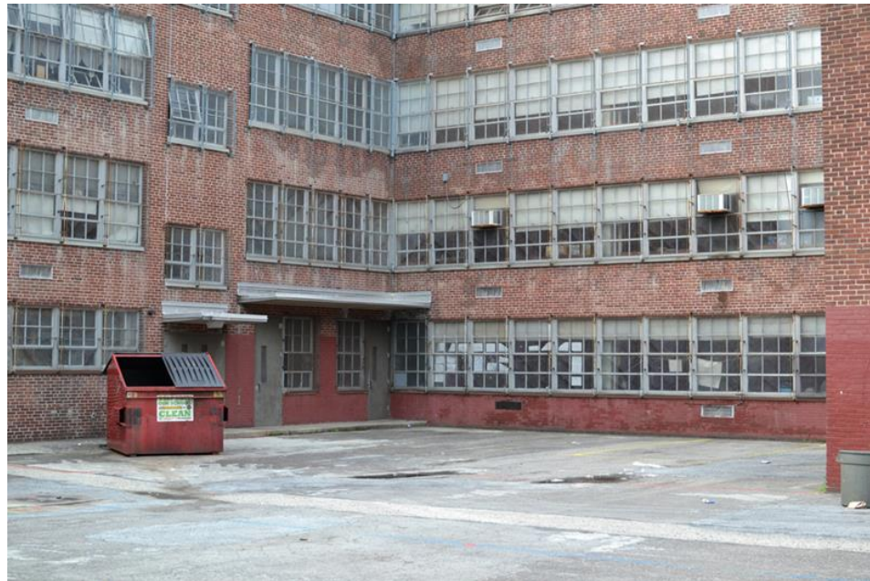
Fig. 4. This grim exterior shot of Alexander Wilson Elementary School was photographed prior to the end of the school year, while the school was still open and in use (June 2013). Photo credit: Steve Minicola, Philadelphia School Closing Photo Collective member.
